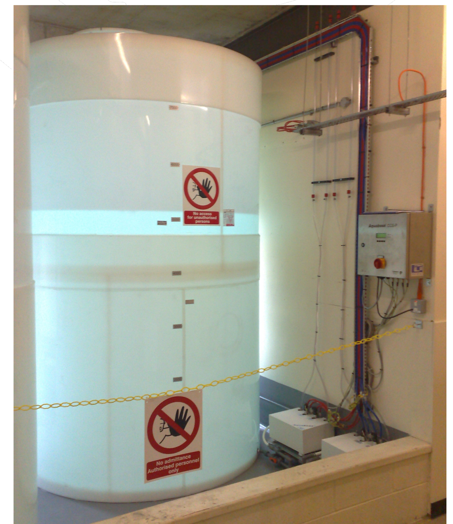
Bulk acid storage tanks in Bradford St Luke's Renal Unit. The central delivery system is saving 16 tonnes CO 2 e and £23,000 per year in reduced acid wastage and reduced plastic waste.
